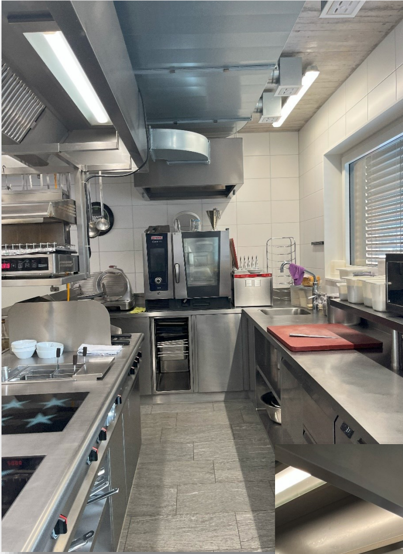
Professional Gourmet Kitchen with the most modern equipment to date
